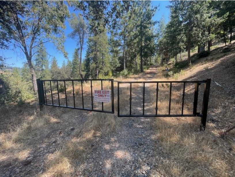
Bottom gate not locked
